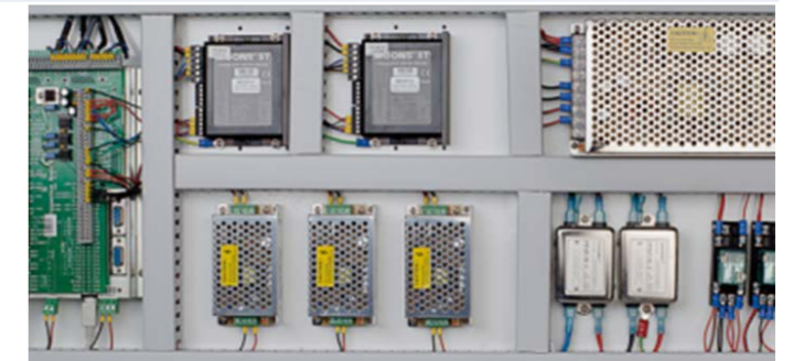
Electrical components of international famous brands
